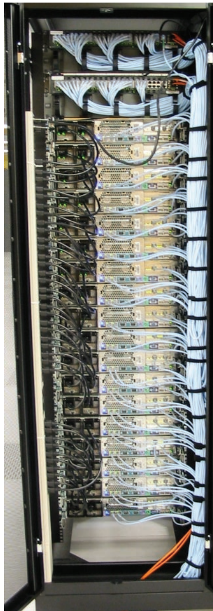
FIGURE 1: TOP OF RACK INTER-CABINET CABLING
