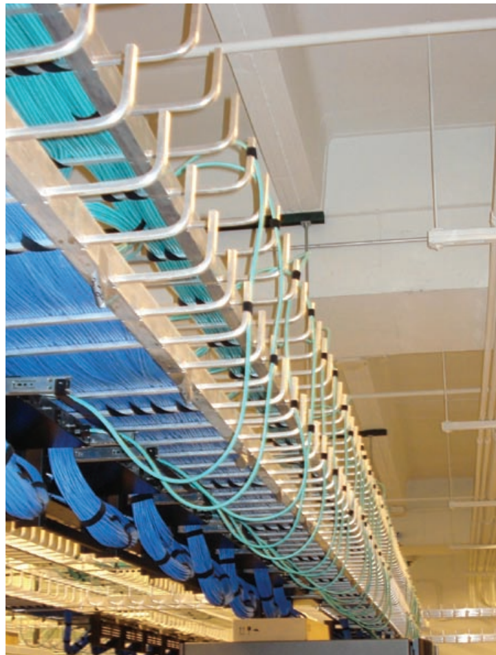
FIGURE 5: STRUCTURED CABLES IN OVERHEAD SPACE
