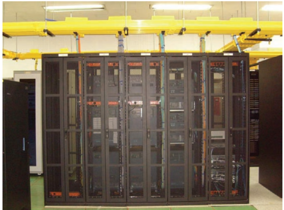
FIGURE 4: THE HDA OF A MEDIA COMPANY'S DATA CENTER
