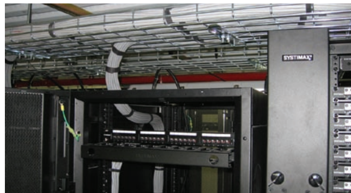
FIGURE 8: SERVER CABINETS OF AN IT SERVICE COMPANY
